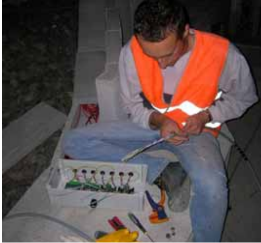
Cable wiring inside Junction Box
